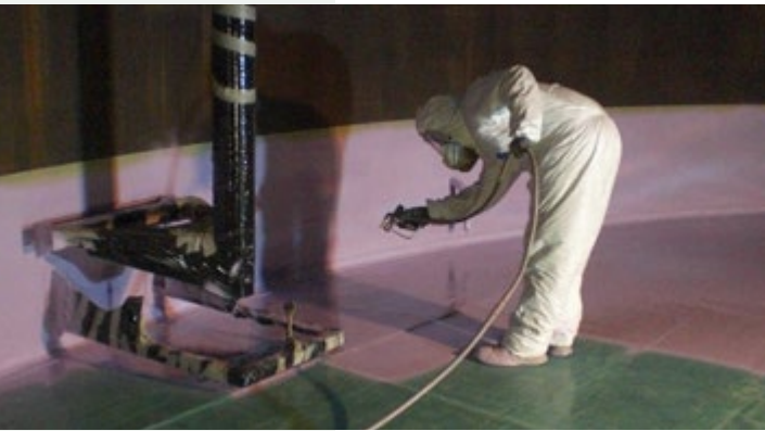
DOPA® system application by Wolftank technicians.
