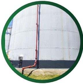
DOPA® double floor refurbishment and ringwall sealing of aboveground storage container in Taiwan.
