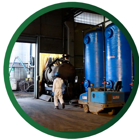
Waste water treatment tanks in Rimini, Wolf tank Rovereta.
