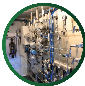
The inside of our Wolftank Hydrogen Smart Container (HSC).
