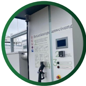
Wolftank Hydrogen Smart Fueller (HSF) installed in Austria.
