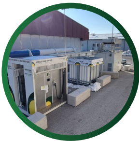
The Multi Hydrogen Fueling Station (MUHF) installed in Villach, Austria to refill local buses.
