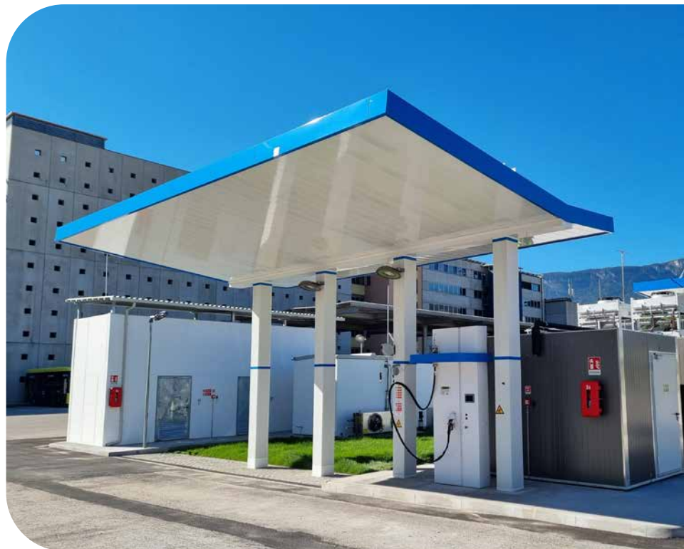
Hydrogen Refuelling Station (HRS) realised for SASA Bolzano
