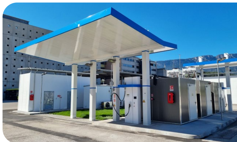
Hydrogen refuelling station developed in Bolzano (Italy).
