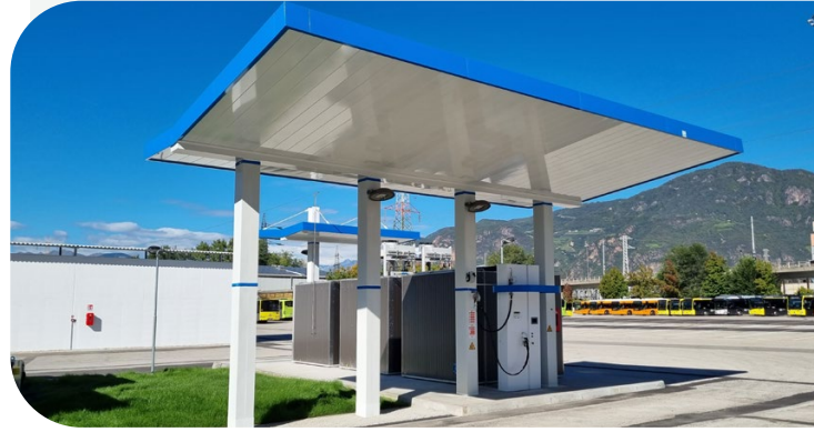
Hydrogen Refuelling Stations (standard, medium and high)
